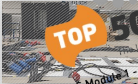
JUWELS Cluster installation begins
